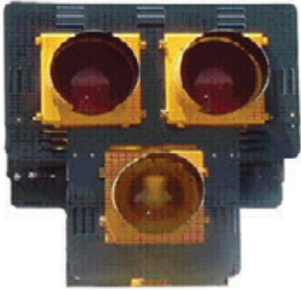
Dark The PHB remains DARK for traffic unless a pedestrian activates the push-button.
